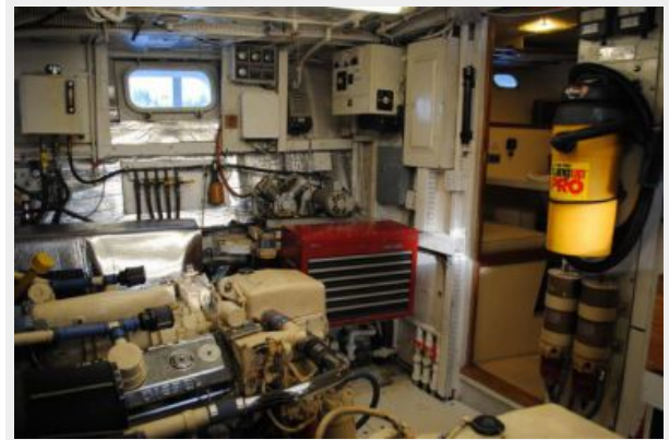
Engine Room Fwd Port
