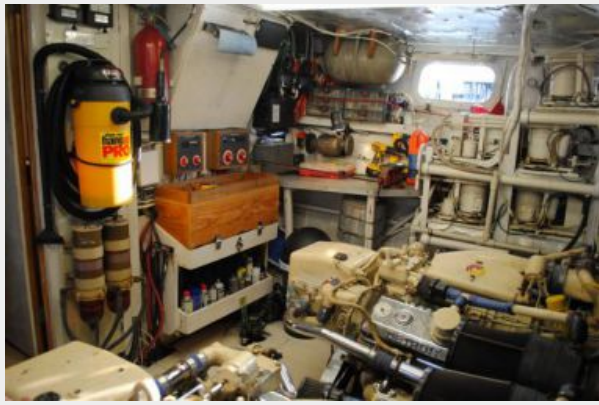
Engine Room Fwd Stbd
