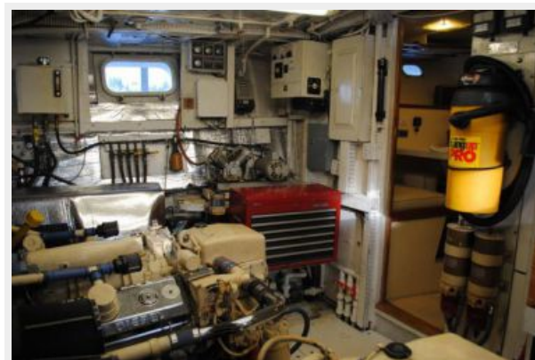
Engine Room Fwd Port
