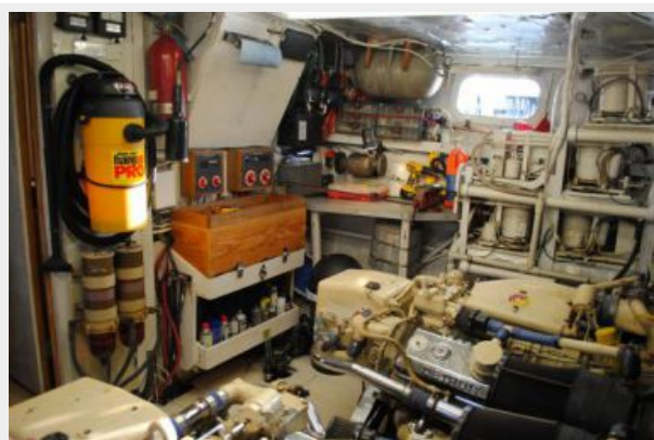
Engine Room Fwd Stbd
