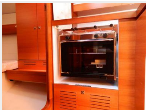
Galley stove with oven
