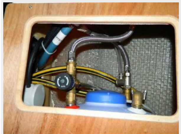
Hot water tank
