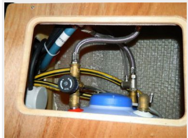
Hot water tank
