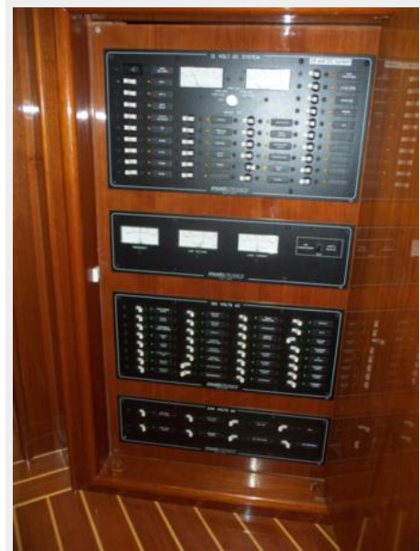
Galley Electrical Panel
