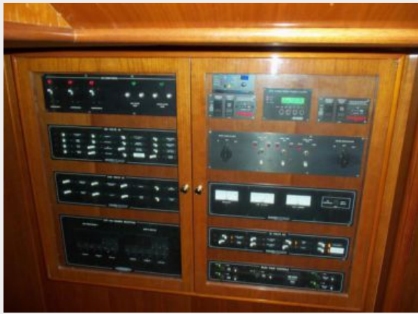
Crew Electrical Panel
