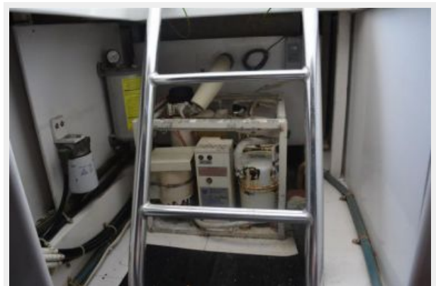
ER access ladder and Eskimo 600 lb icemaker
