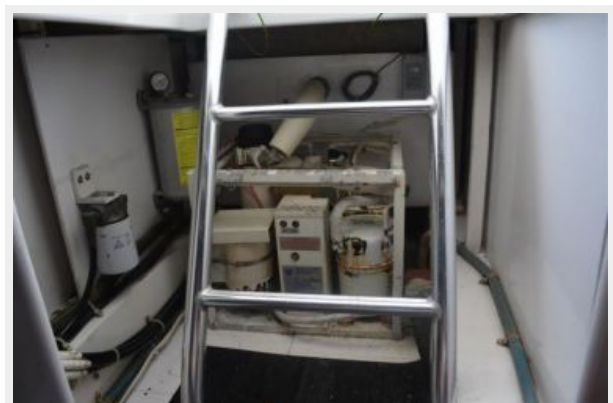
ER access ladder and Eskimo 600 lb icemaker
