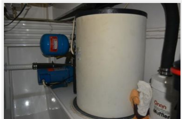
water heater on generator shelf
