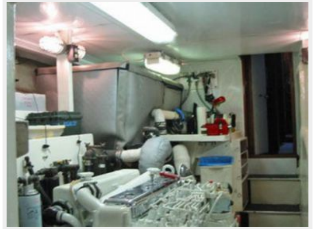
Walkin Engine Room
