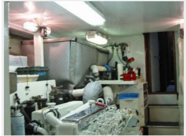
Walkin Engine Room
