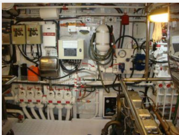
97' Santa Margherita engine room forward
