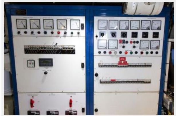
97' Santa Margherita engine room electrical panels
