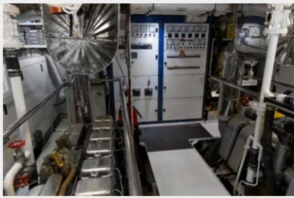
97' Santa Margherita engine room aft
