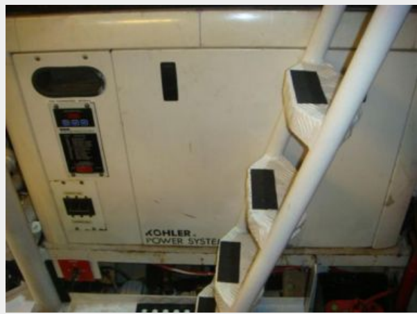
97' Santa Margherita night generator
