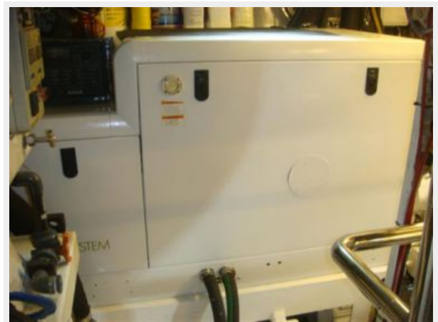
97' Santa Margherita port generator sound box
