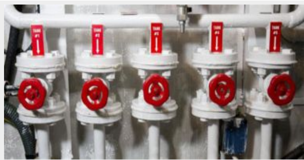
97' Santa Margherita fuel manifold
