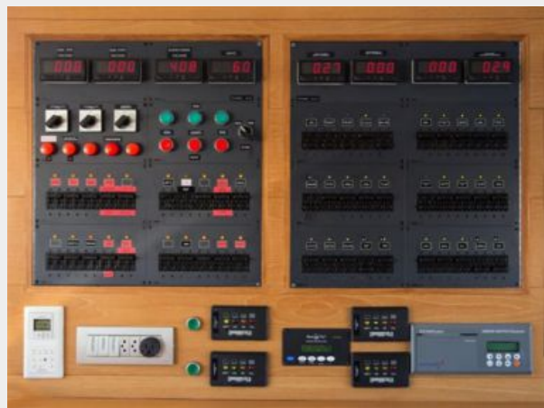
97' Santa Margherita pilothouse electrical panel
