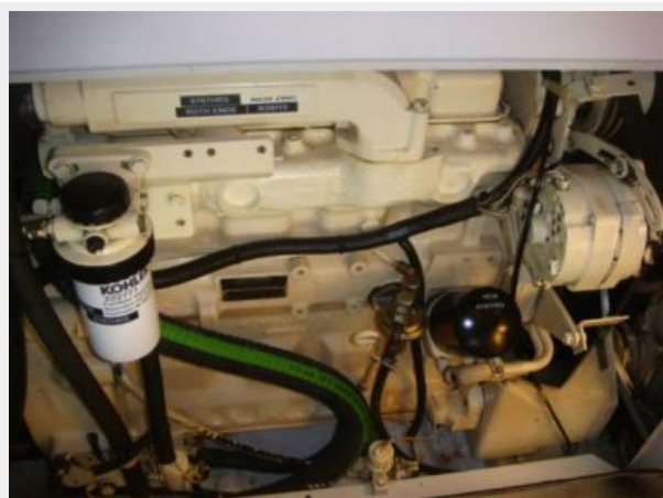
97' Santa Margherita port generator
