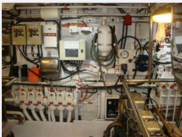
97' Santa Margherita engine room forward
