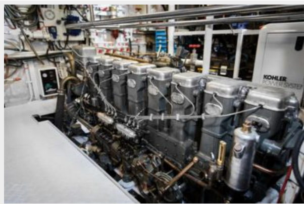
97' Santa Margherita starboard main engine photo1
