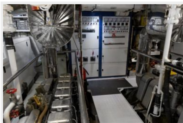
97' Santa Margherita engine room aft
