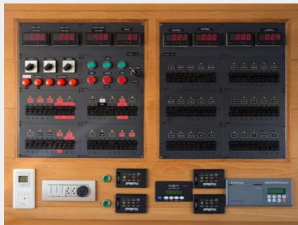
97' Santa Margherita pilothouse electrical panel
