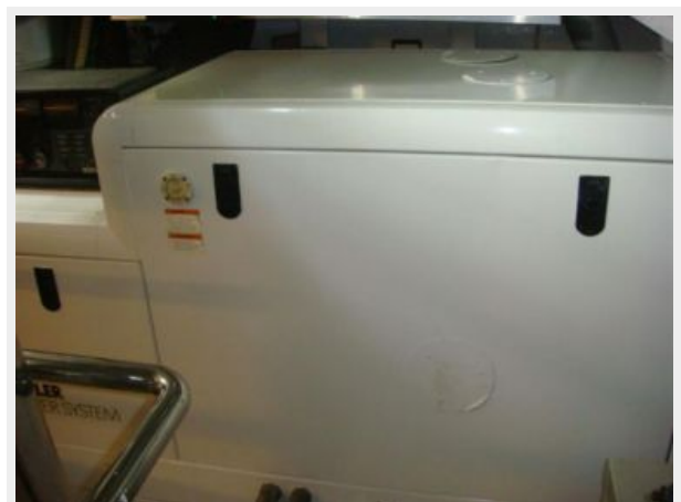
97' Santa Margherita starboard generator sound box
