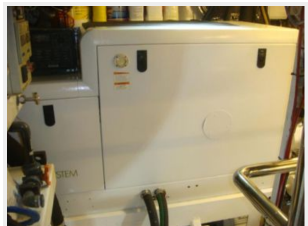
97' Santa Margherita port generator sound box
