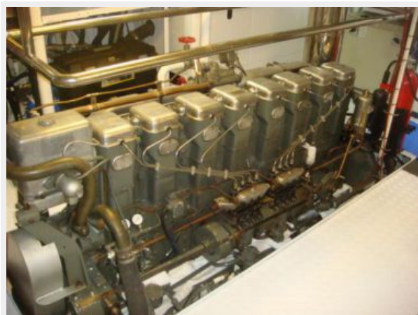
97' Santa Margherita starboard main engine photo2
