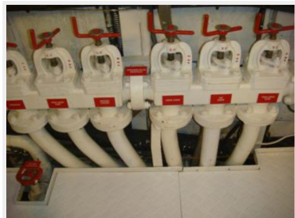
97' Santa Margherita bilge manifold
