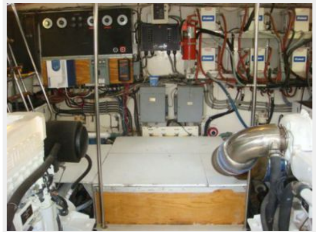
64' Hatteras engine room forward
