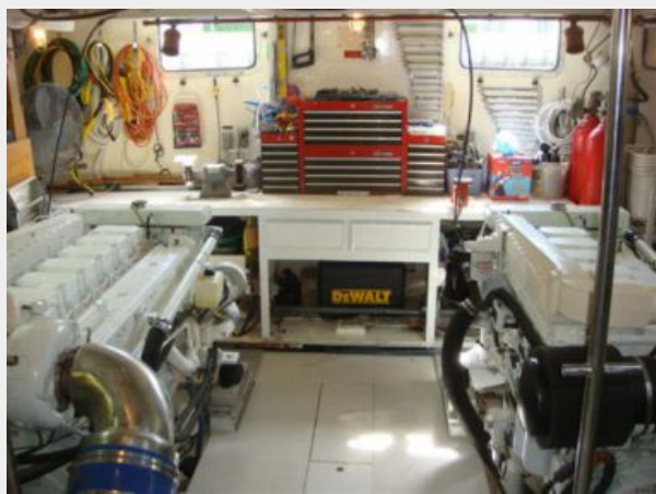
64' Hatteras engine room aft
