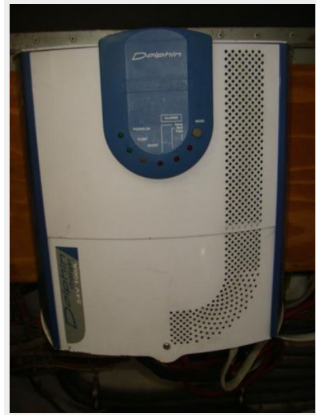
64' Hatteras battery charger2
