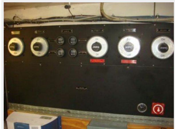
64' Hatteras battery switches
