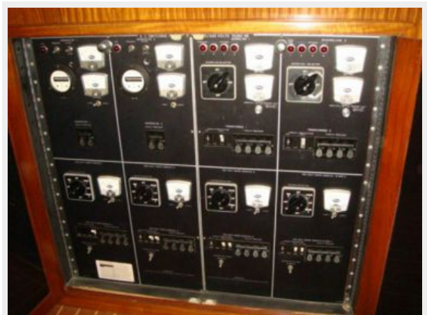
64' Hatteras electrical panel
