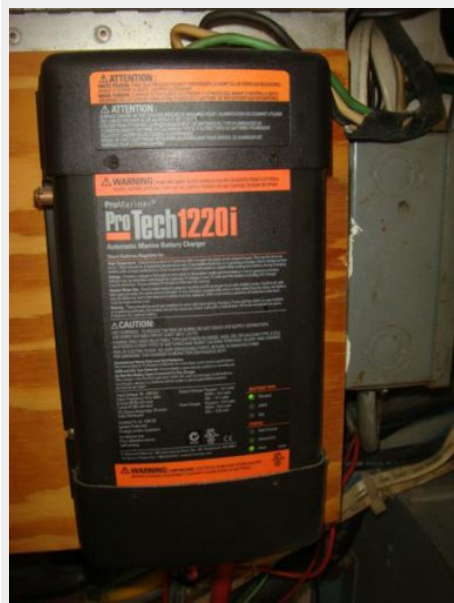
64' Hatteras battery charger3
