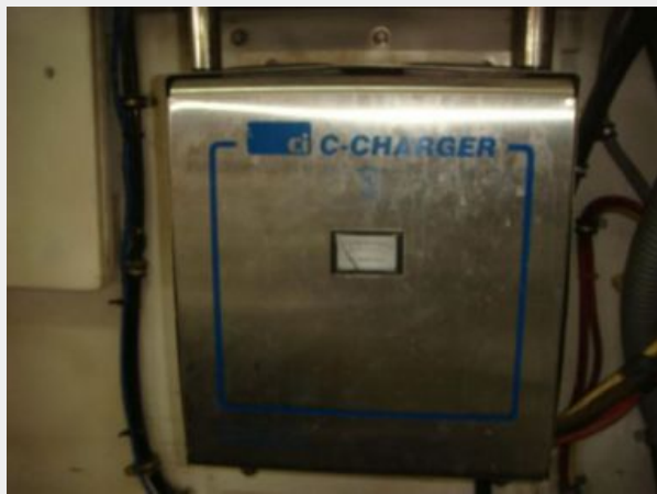
64' Hatteras battery charger1
