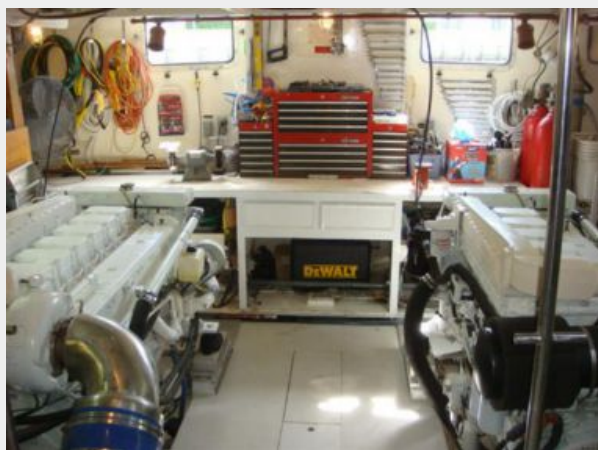
64' Hatteras engine room aft
