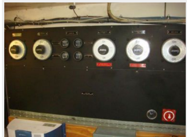
64' Hatteras battery switches
