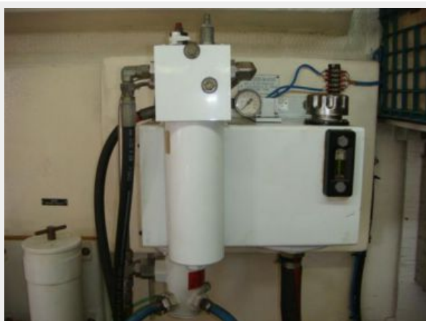
64' Hatteras stabilizer system
