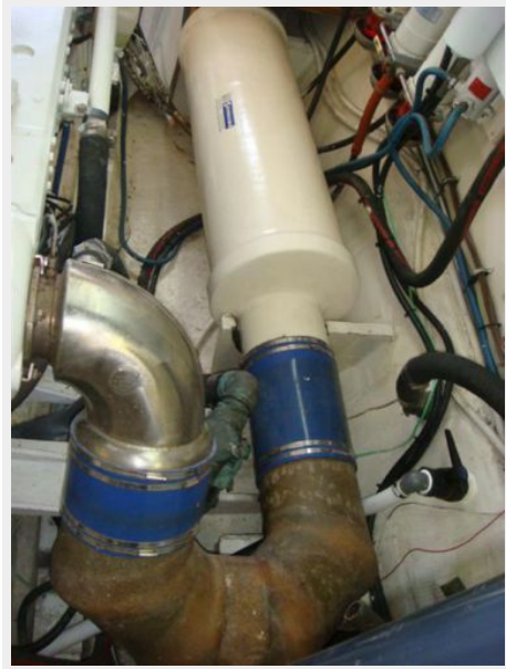
64' Hatteras port main engine exhaust
