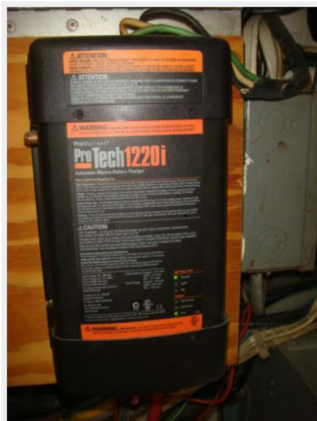
64' Hatteras battery charger3
