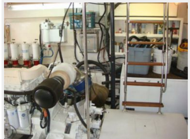
64' Hatteras engine room port
