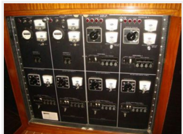
64' Hatteras electrical panel
