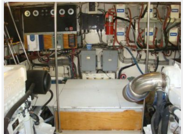
64' Hatteras engine room forward
