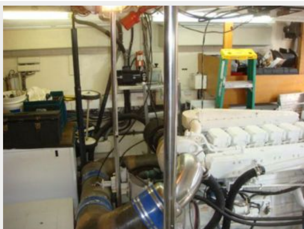
64' Hatteras engine room starboard
