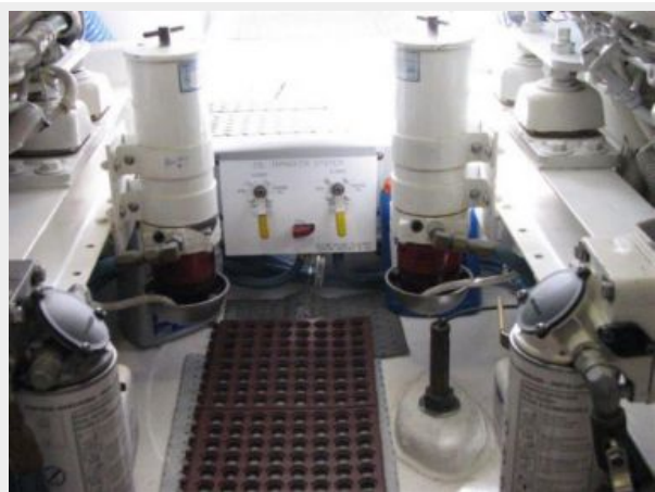
Engine & Mechanical Equipment 5
