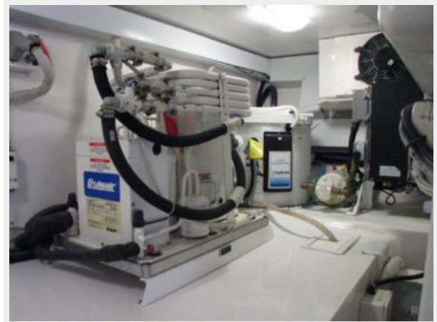
Engine & Mechanical Equipment 4
