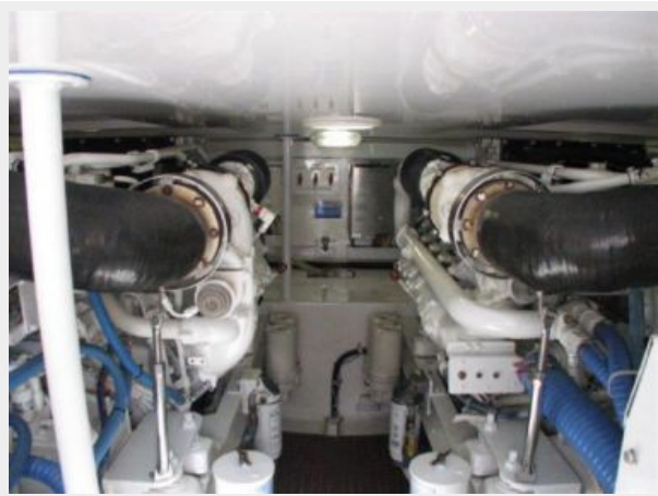
Engine & Mechanical Equipment 1 - Engine Room
