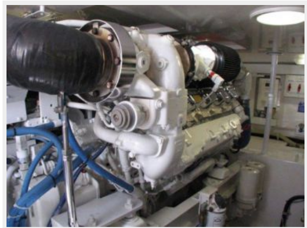
Engine & Mechanical Equipment 2 - Port Engine
