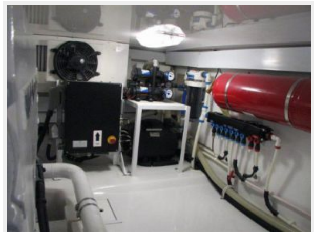
Engine & Mechanical Equipment 6
