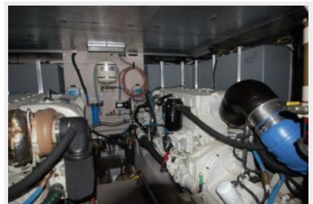
Twin Cummins QSM11 Diesels - Less than 300 hours
