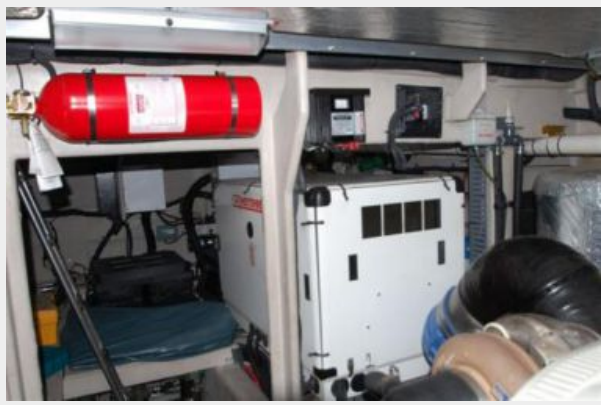
Westerbeke generator - Gen set in sound shield
