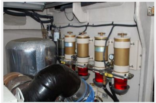
Racor fuel filter system - Dual Racor 1000 system's
