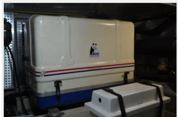
49' Krogen Express generator
