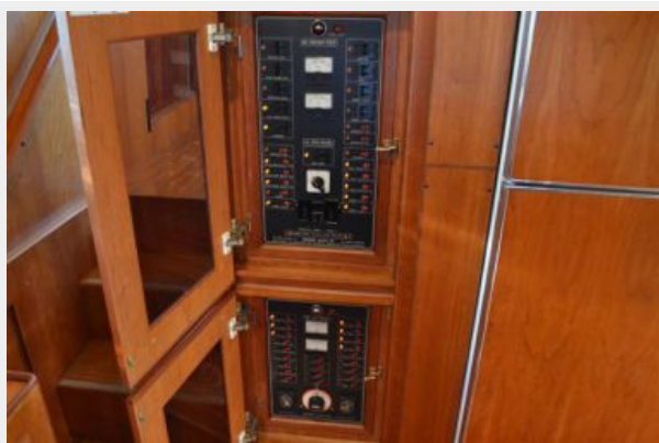
49' Krogen Express electrical panel
