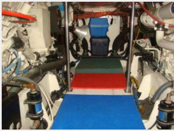
47' Bayliner engine room aft
