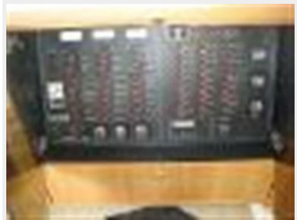
47' Bayliner electrical panel
