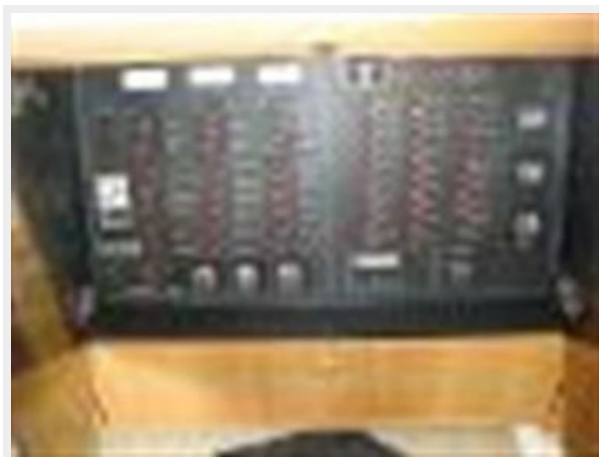
47' Bayliner electrical panel
