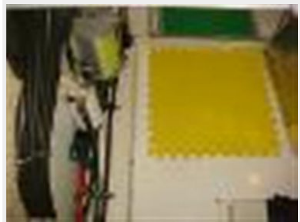
47' Bayliner engine room access
