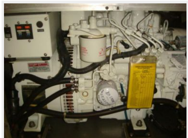
34' American Tug generator
