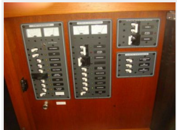
34' American Tug electrical
