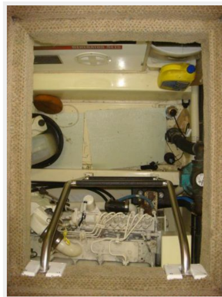
34' American Tug engine room access
