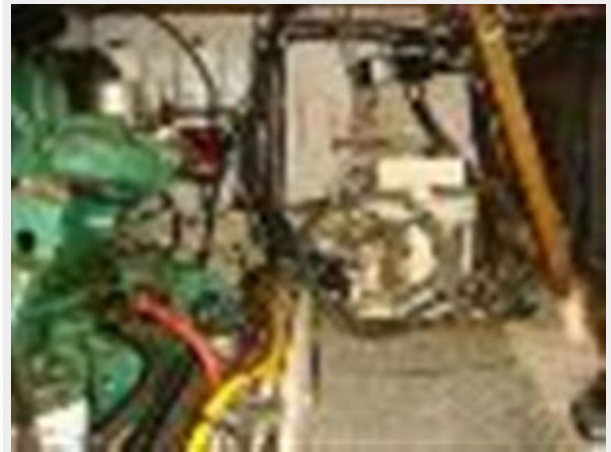
36' CT Trawler engine room port aft
