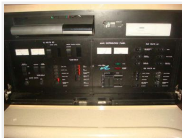
45' Sea Ray electrical panel
