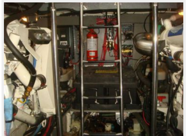
45' Sea Ray engine room aft
