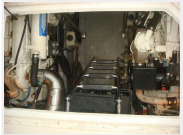
45' Sea Ray engine room access
