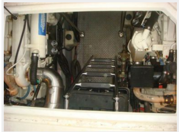
45' Sea Ray engine room access
