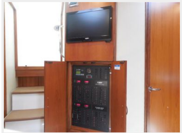
Salon TV and breaker panel
