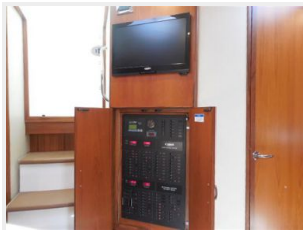
Salon TV and breaker panel
