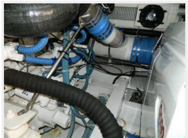
Engine & Mechanical Equipment 2
