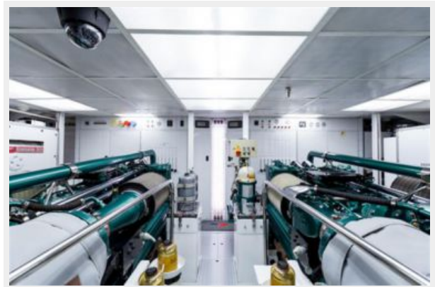
Engine Room Forward View
