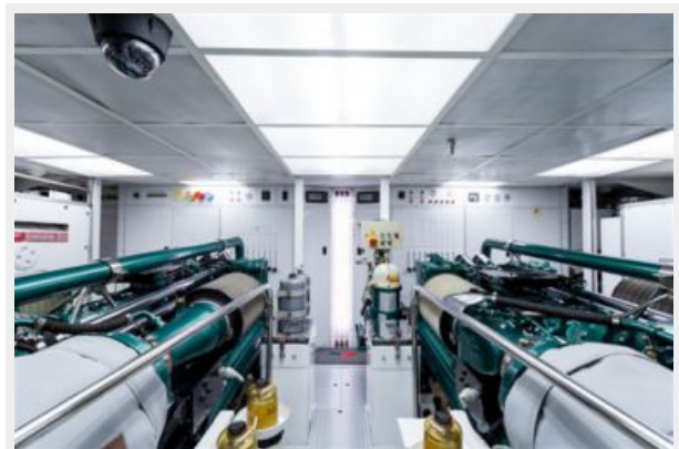
Engine Room Forward View
