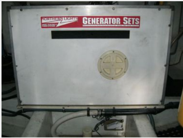
Northern Lights Generator
