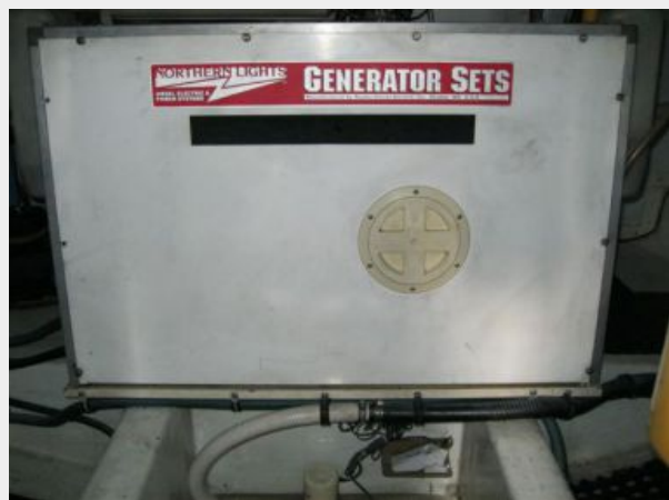
Northern Lights Generator
