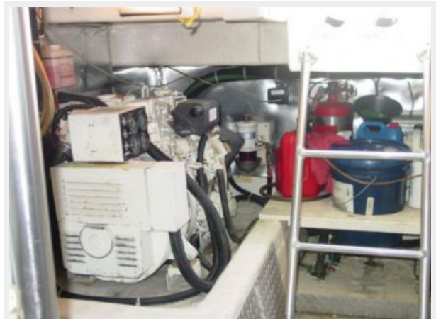
Engine & Mechanical Equipment 3
