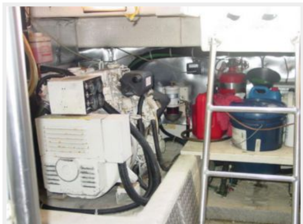
Engine & Mechanical Equipment 3
