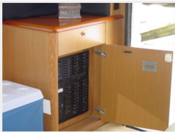
Salon 8 - Electric Breaker Panel
