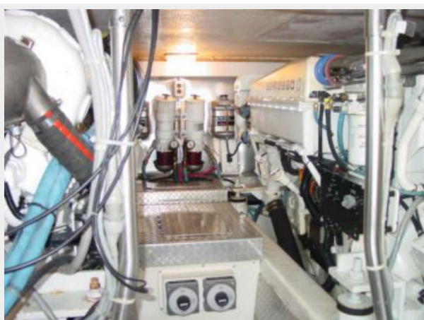
Engine & Mechanical Equipment 2
