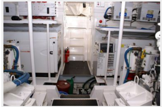
Engine Room Entry & Generators
