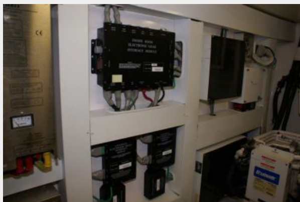
Engine Control Interface
