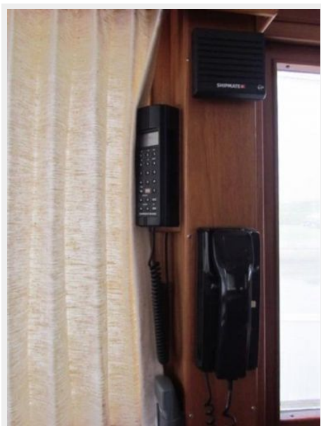
Lower Helm VHF, VHF Speaker, Intercom
