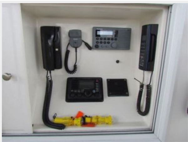
Electronics Cabinet next to upper helm
