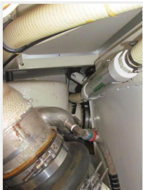
Engine Room off Set Fuel Fill Starboard
