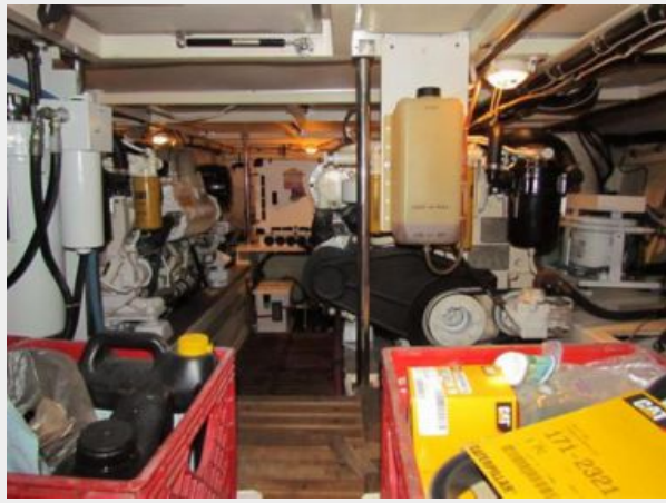
Engine Room Looking Aft
