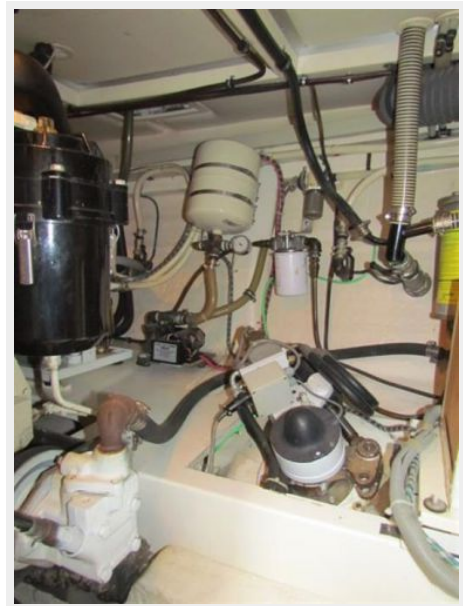
Engine Room Starboard Stabilizer
