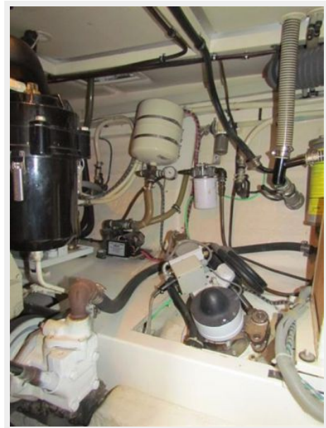
Engine Room Starboard Stabilizer
