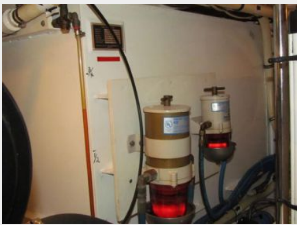
Engine Room Starboard Fuel Tank
