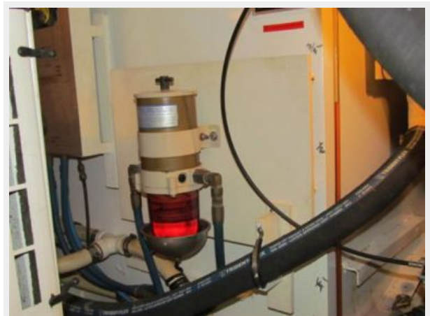
Enginr Room Port Fuel Tank
