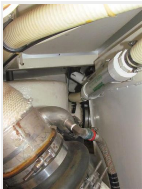
Engine Room off Set Fuel Fill Starboard
