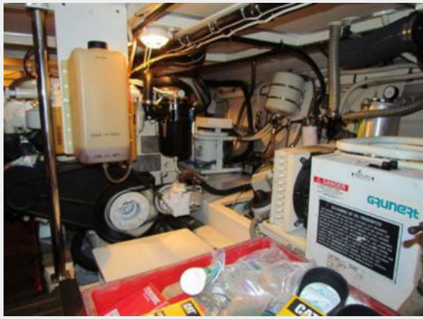
Engine Room Port
