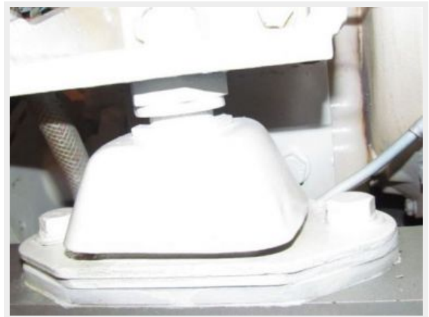
Engine Room Motor Mount
