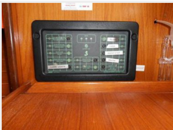
Electrical Panel at Nav Station
