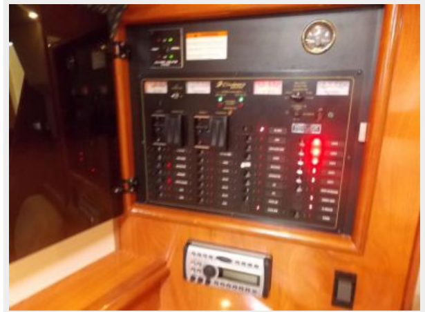
Main Distribution Panel
