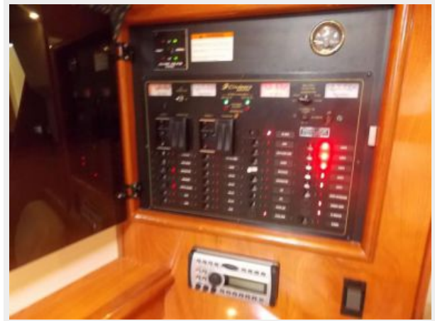
Main Distribution Panel
