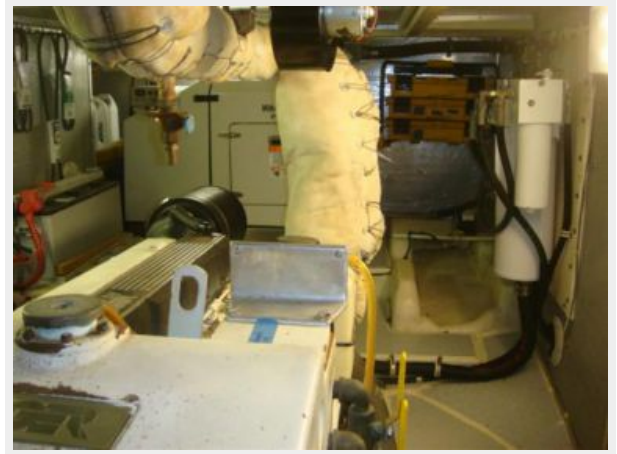
40' Nordhavn engine room aft
