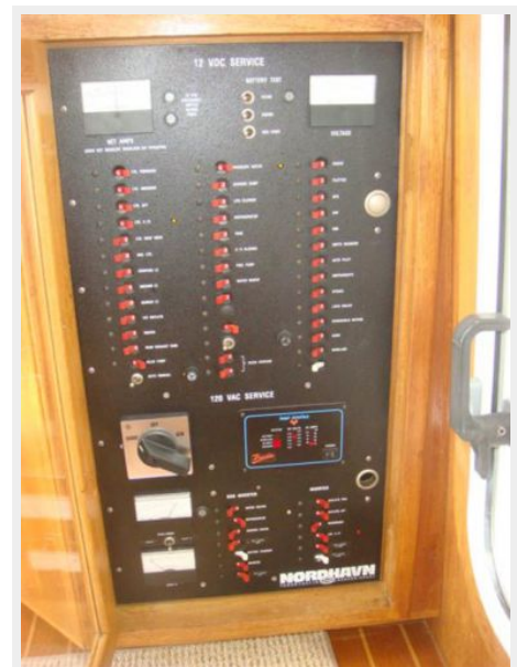
40' Nordhavn electrical panel
