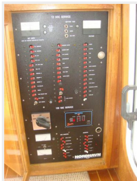
40' Nordhavn electrical panel
