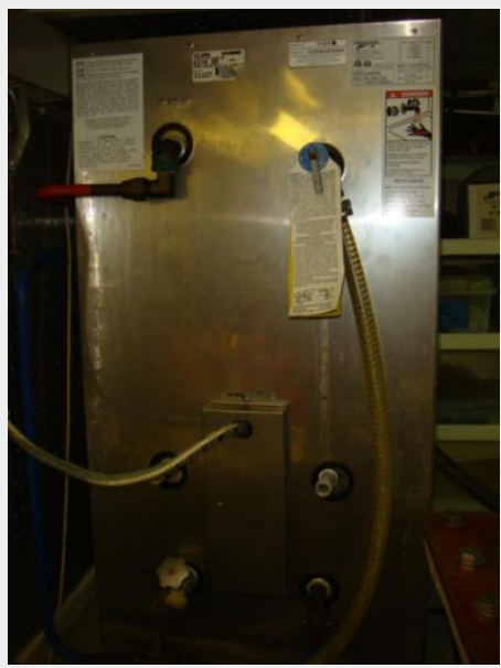
49' DeFever water heater
