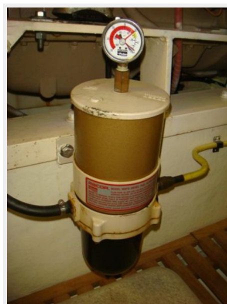
49' DeFever starboard Racor fuel filter
