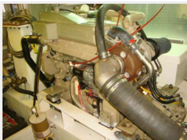
49' DeFever starboard main engine photo2
