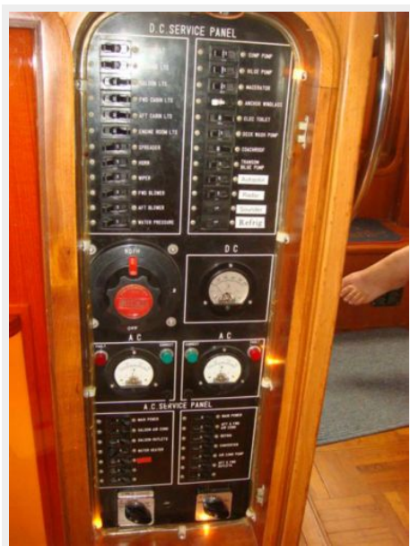
42' Jefferson electrical panel
