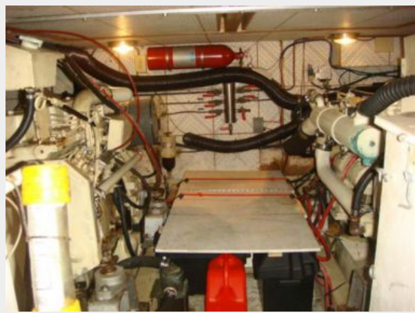
42' Jefferson engine room aft
