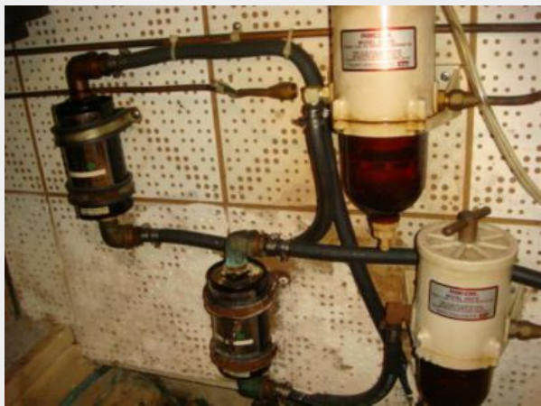
42' Jefferson fuel polishing system
