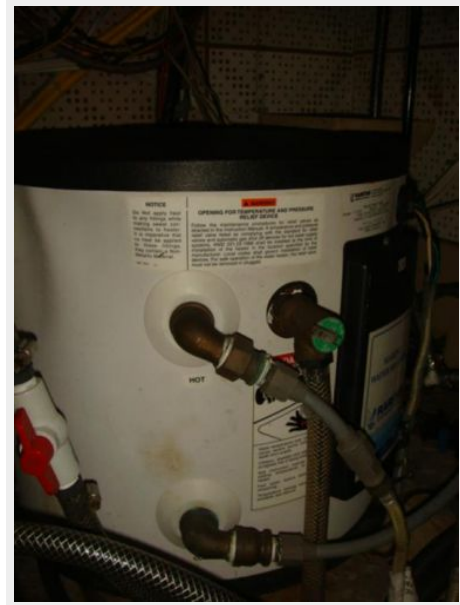
42' Jefferson water heater
