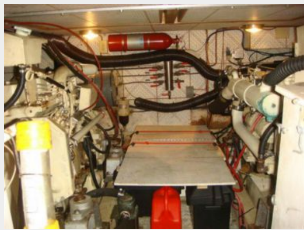
42' Jefferson engine room aft
