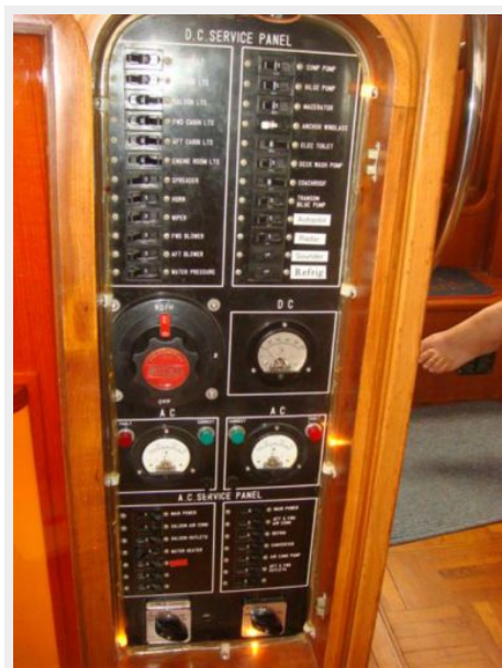
42' Jefferson electrical panel
