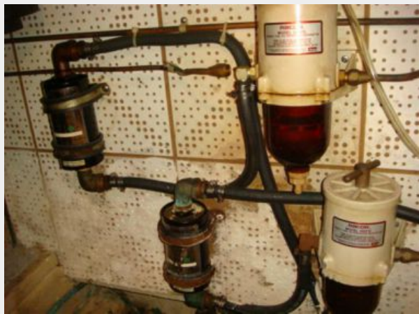
42' Jefferson fuel polishing system
