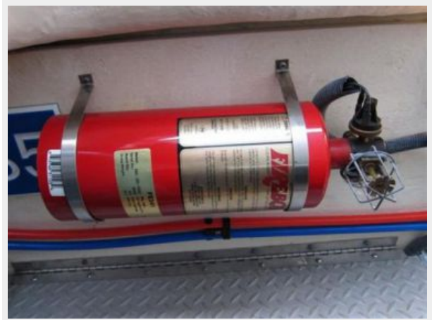
Fire Suppressant system
