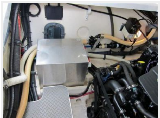
Spotless Engine room
