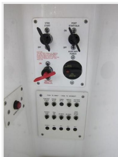
Battery switches, Fuses
