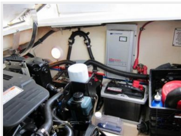
Spotless Engine room
