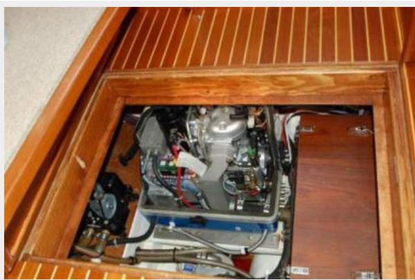
Fisher Panda Generator - Portion of sound shield is removed
