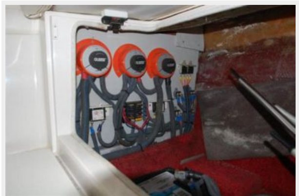
Electrical Battery Switches - Under port cockpit seating.
