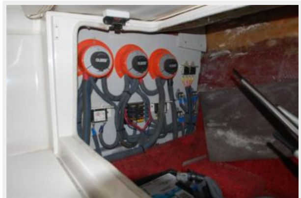
Electrical Battery Switches - Under port cockpit seating.
